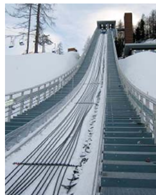
Figure 2.57 - Cooling serpentine along the LH ramp
