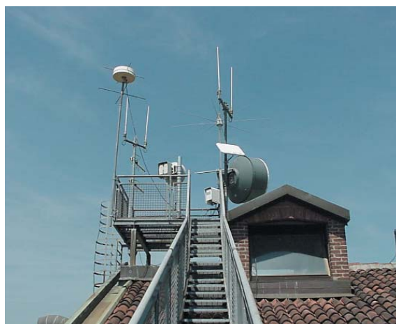
Figure 2.183 - The portable automatic weather station installed on the roof of the WOC office
